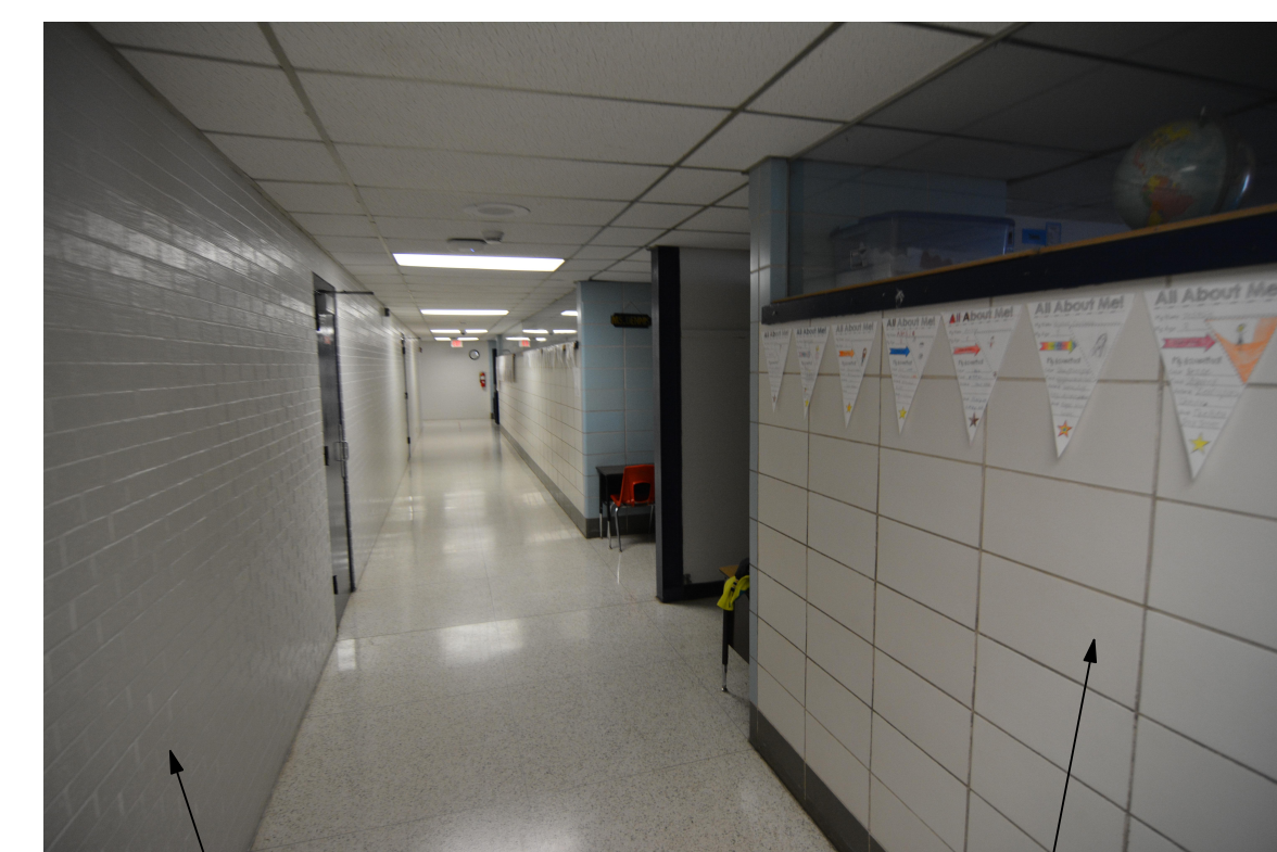
CORRIDOR WALLS, INTERIOR CORE: EXPOSED BRICK CORRIDOR WALLS, OUTSIDE PERIMETER: TILE OVER CMU. SEE BID ALTERNATE #5.
